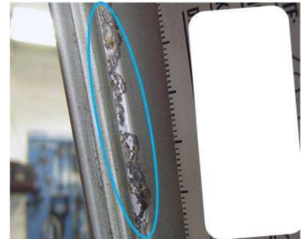
Blisters burst open without external influence and red rust becomes visible. In this case, width of blisters is not longer main criteria.
