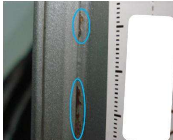
Blisters burst open without external influence and red rust becomes visible. In this case, width of blisters is not longer main criteria.
