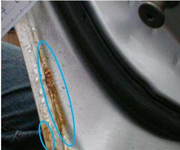
Blisters burst open without external influence and red rust becomes visible. In this case, width of blisters is not longer main criteria.
