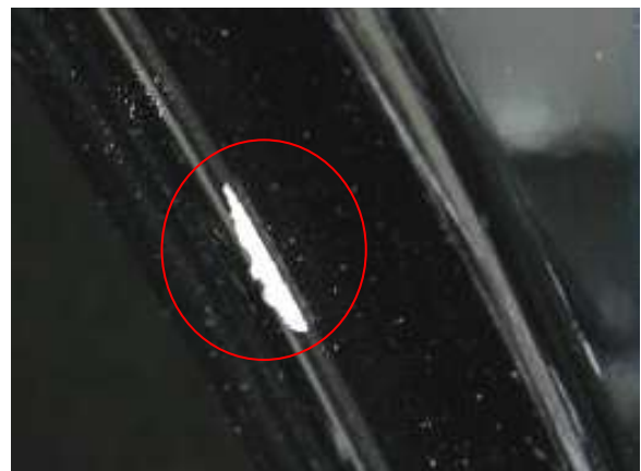
Paint damage only
