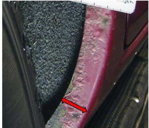
Visible blisters and red rust in an area more than 10mm from the inner edge of the wheel arch.
