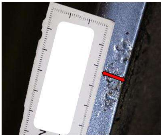
Visible blisters in an area more than 10mm from the inner edge of the wheel arch.
