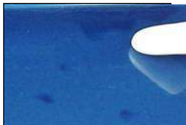
Due to high temperature under the sun, acid in the waterdrop penetrated into the paint coating, damaging aluminum pieces.
