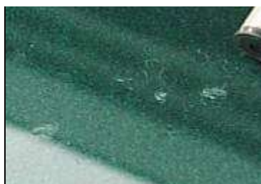
Trace of the paint surface etched off by acid because waterdrops were left under the scorching sun.
