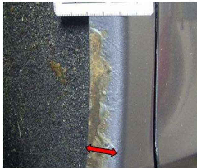
Visible blisters and red rust in an area more than 10mm from the inner edge of the wheel arch.
